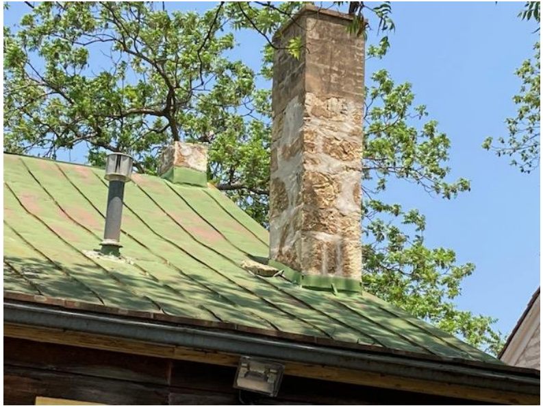
Figure 5 Chimneys after caps were blown off. Part of chimney crown is resting on roof.
