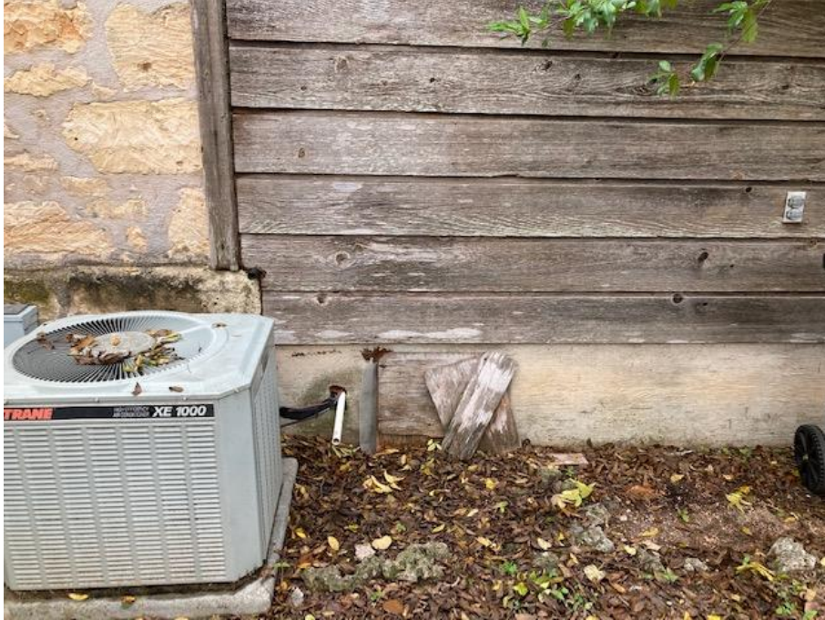
Figure 7 Proposed location of water softener next to air conditioner compressor.
