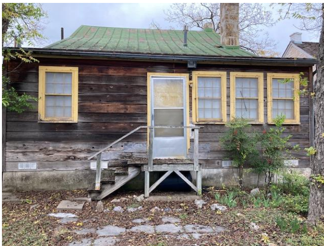
Figure 6 Back of house showing back door landing and steps to be replaced with deck.
