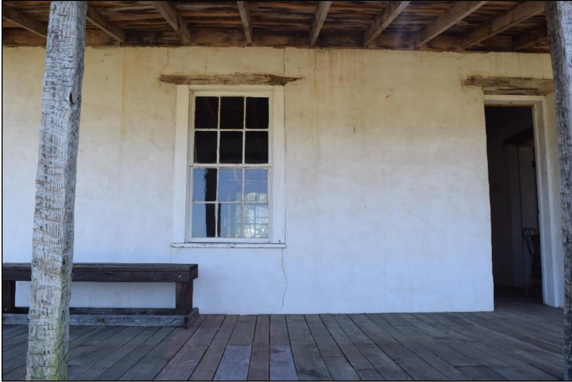
Figure B-19. Structural cracks around window on the southwest side of Building E, facing northeast.
