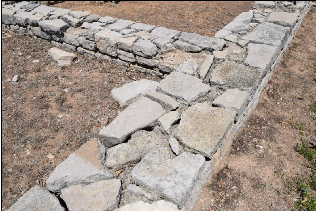
Figure B-23. Mortar loss and minor stone displacement in stabilized foundation of Building G.
