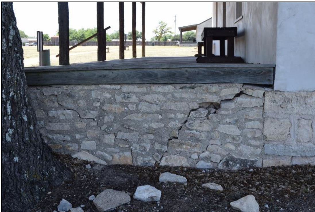
Figure B-20. Structural cracks in porch foundation of Building E, caused by tree root growth. Facing northwest.
