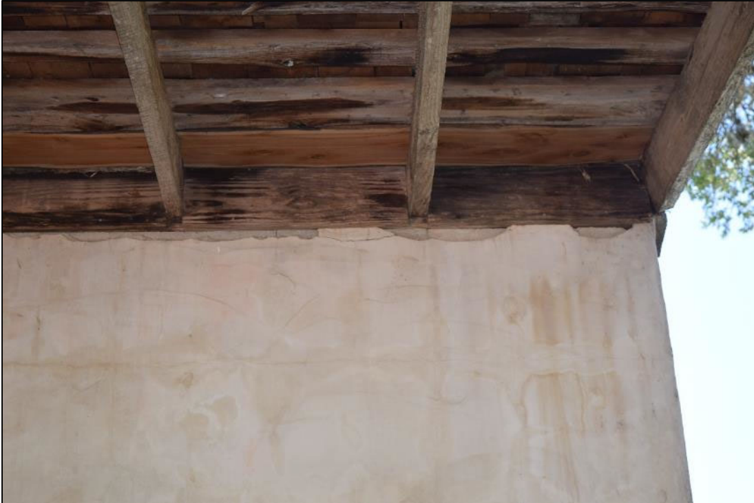
Figure B-21. Minor cracking and loss of concrete stucco at wall top of Building E, facing northeast.
