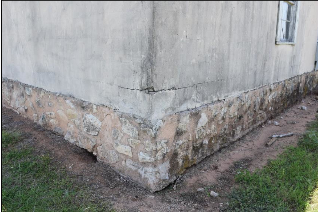
Figure B-15. Detail of deterioration conditions at northeast corner of Building B. Note major horizontal cracks, fine cracks in stucco along concrete block wall joints, and animal burrow at bottom left.
