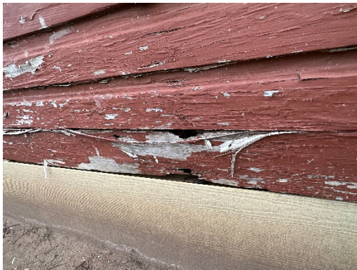
West side of house rot
