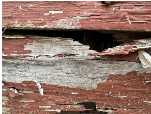
West side of house rot
