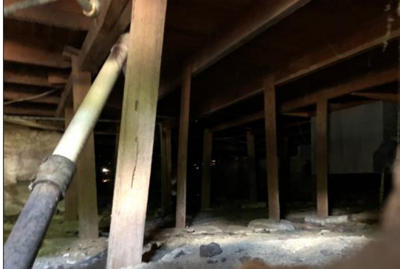
Existing pier beam floor framing has limited and inadequate support.
