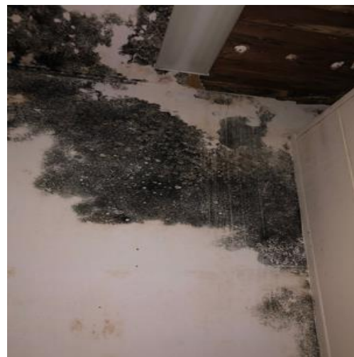
Existing Mold inside of house.
