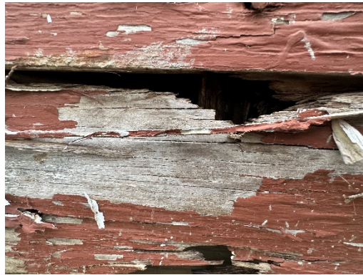
West side of house rot
