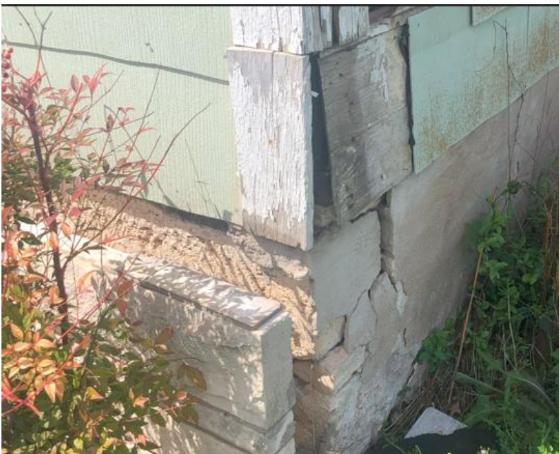
Corner foundation & wall failure
