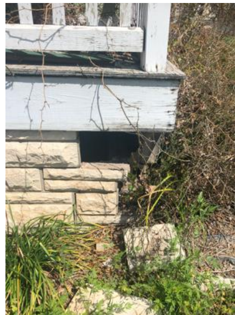
Porch foundation failure.
