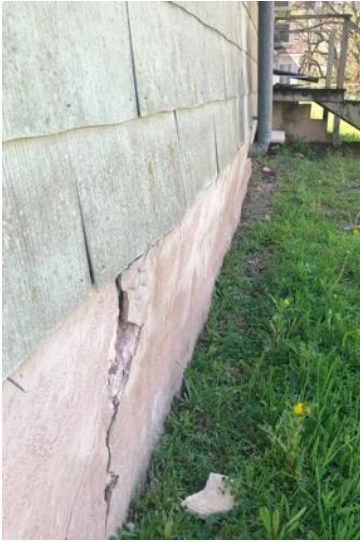
North foundation wall failure
