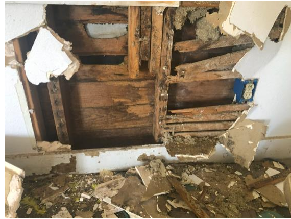
Typical interior wall framing & siding failure.
