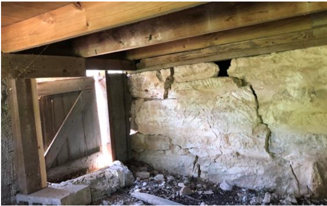
Stone perimeter wall is compromised.
