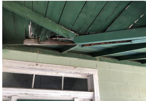
Porch roof framing failure.
