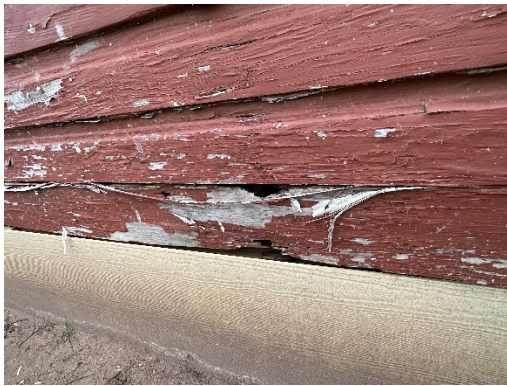
West side of house rot
