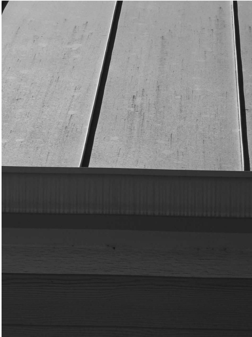
13 13-20240623_152321 Date Taken: 6/23/2024 Hail damage to metal roof
