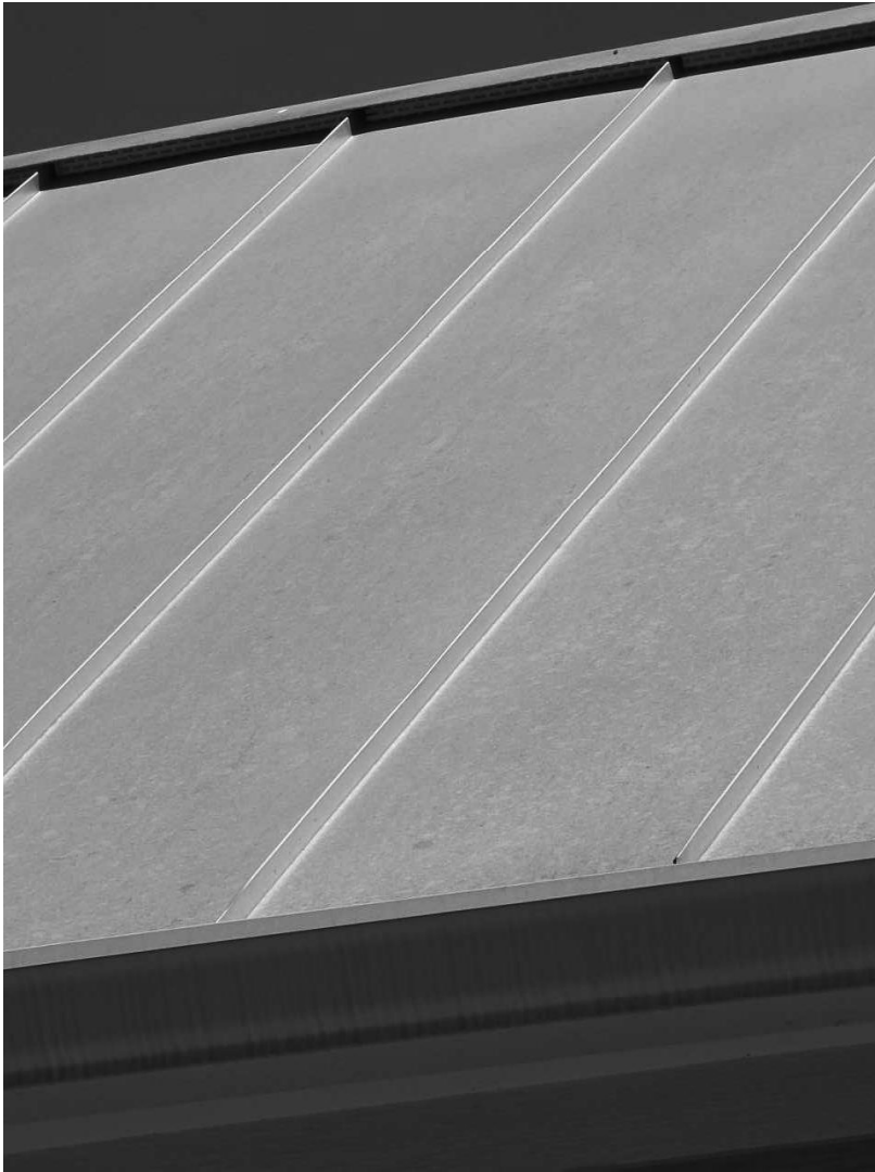
17 17-20240623_152815 Date Taken: 6/23/2024 Hail damage to metal roof
