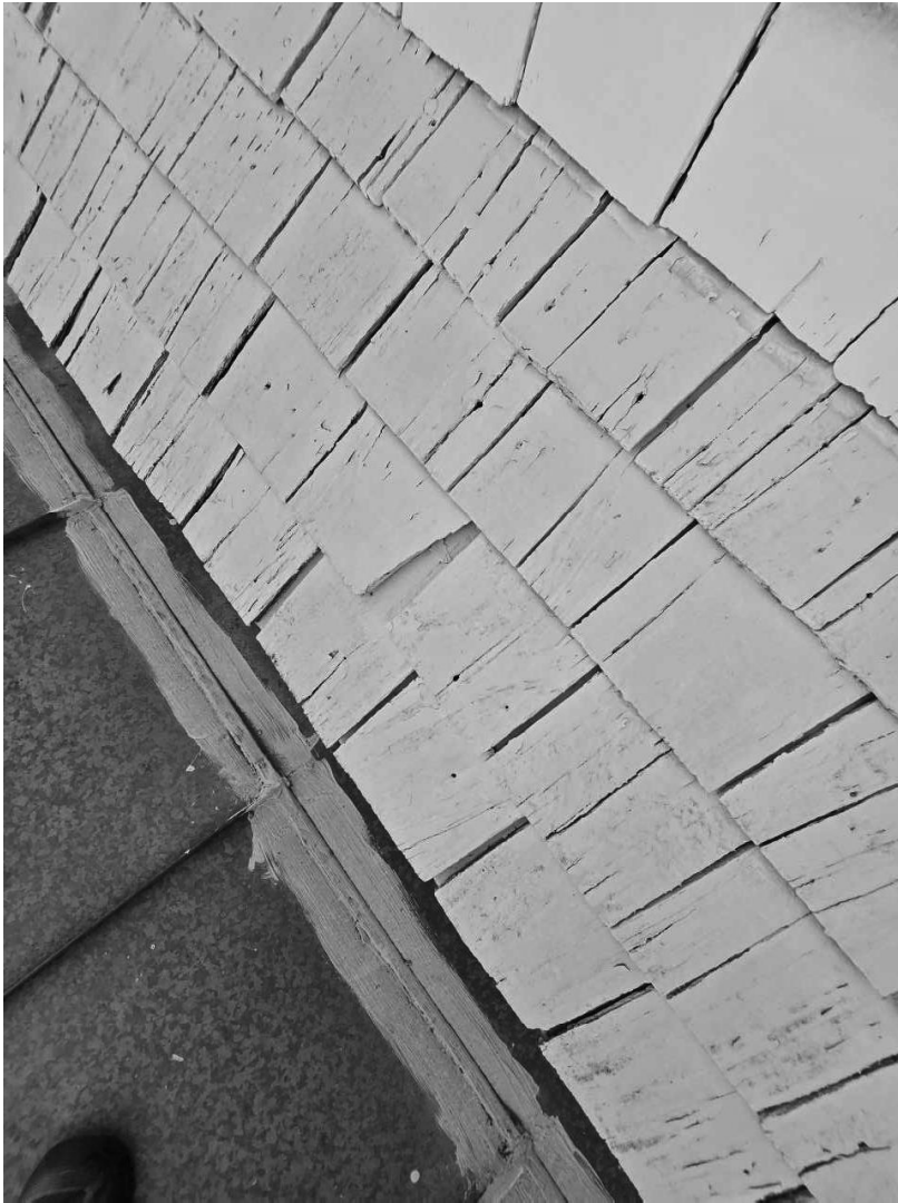
10 10-20240623_151817 Date Taken: 6/23/2024 Hail damage to cedar shake
