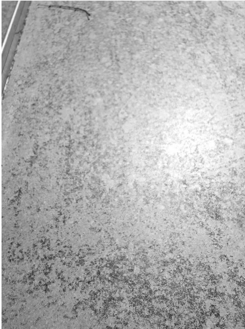
15 15-20240623_152633 Date Taken: 6/23/2024 Hail damage to metal roof
