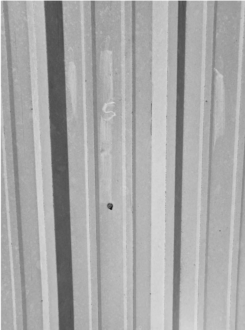
3 3-20240623_151652 Date Taken: 6/23/2024 Hail damage to metal roof
