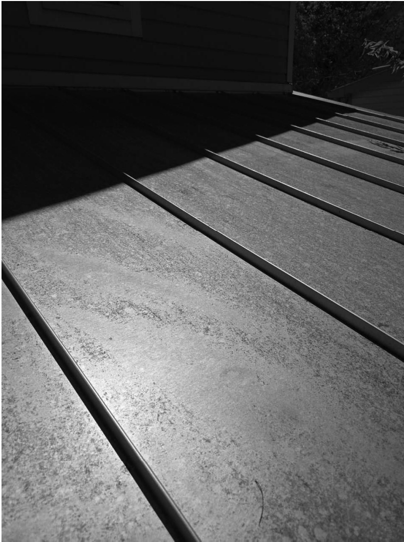
16 16-20240623_152636 Date Taken: 6/23/2024 Hail damage to metal roof
