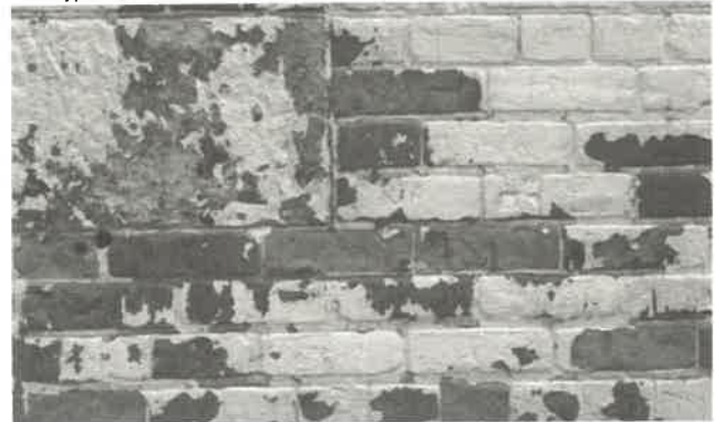
Figure 3-21. Example of damage to brick surface caused by paint. Paint can allow moisture to become trapped within the brick, resulting in flaking off the brick's hard outer crust along with the paint, leaving the softer inner brick exposed and susceptible to weatherization. Source: "Please, Don't Paint Your Mid-Century Brick," MidMod Midwest, accessed January 8, 2021, https://midmod-midwest.com/mid-century-brick/ .
