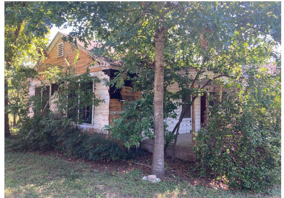
SOUTHWEST ELEVATION. PORCH ON RIGHT TO BE RESOTRED TO ORIGINAL CONDITION
