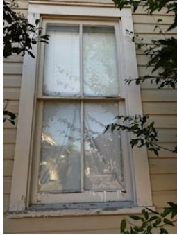
Old window damaged by hail storm and is rotten
