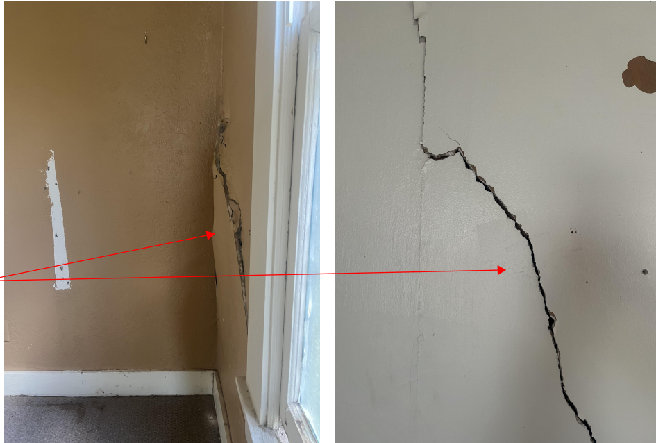
Figures 22 (left) & 23(right): Interior wall buckling at 701 N. Llano (2024)
