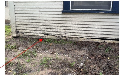
Fig. 10 (top) & 11 (bottom): Damage at North Facade (2024)
