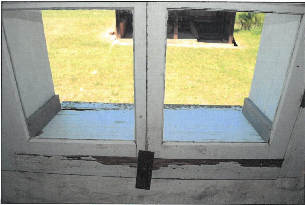
Figure B-33. Wood damage at window sill exterior and interior on north side of Building N, the Guard House.
