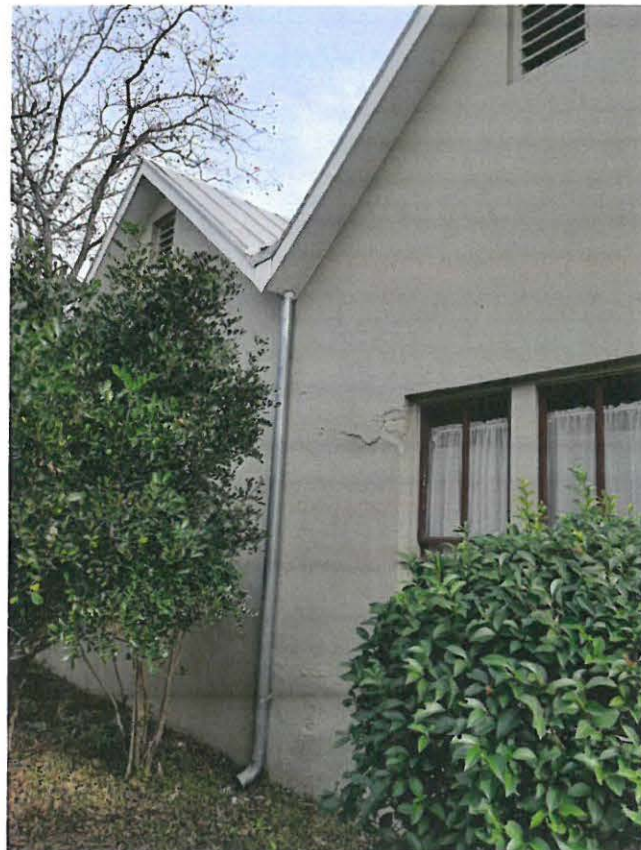
Captive gutter and water damage around windows
