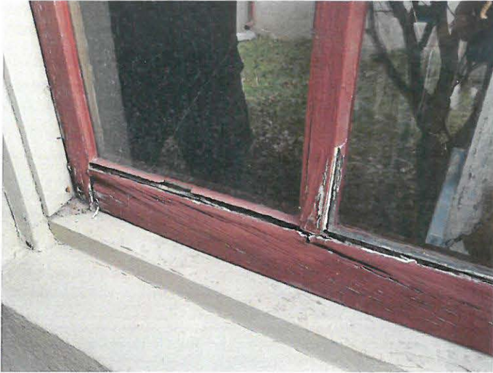
Wood window needs to be replaced.
