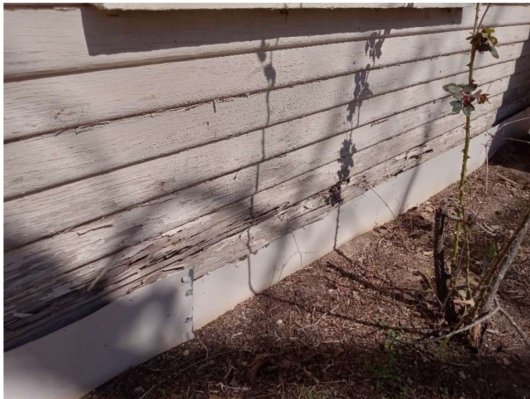
Photo 14 – Siding damaged by rot from ground contact – Garage.
