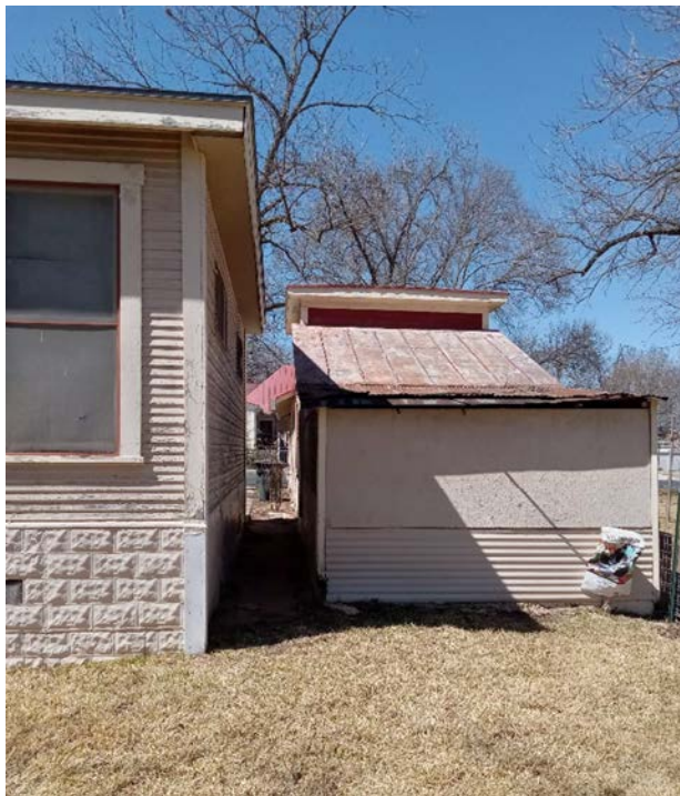
Photo 9 – Sheds 3 ft. from house
