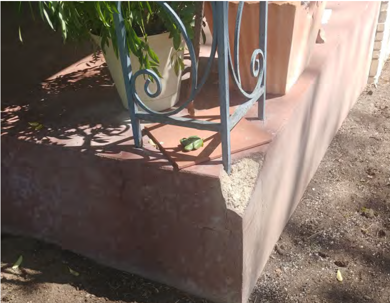
Front porch in need of repair
