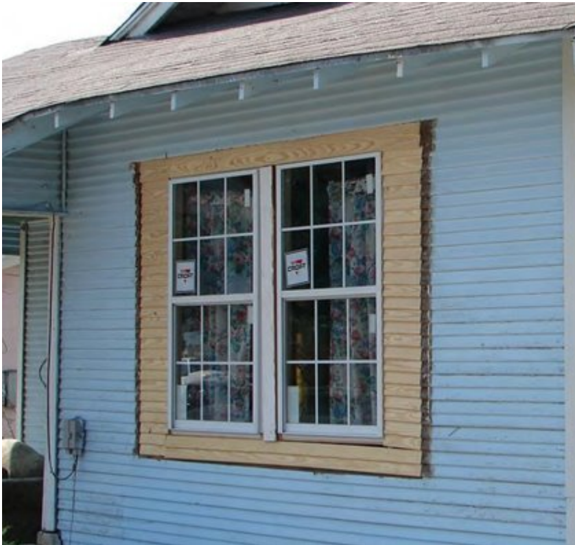
Figure 3-32. Example of inappropriate installation of replacement windows. Source: City of San Antonio Office of Historic Preservation.
